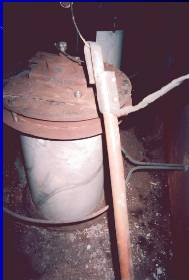
Cracked Support insulator
